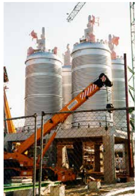
4 reactors 110 m 3 3 stages of GlasLock® agitators
